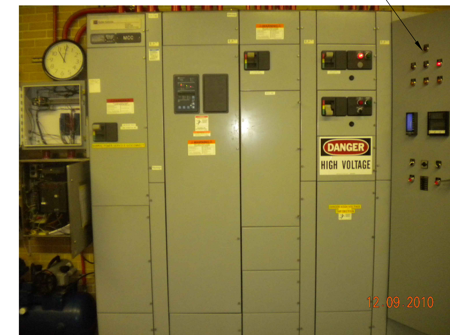
4 EXISTING CONTROL PANEL SCALE: NOT TO SCALE
