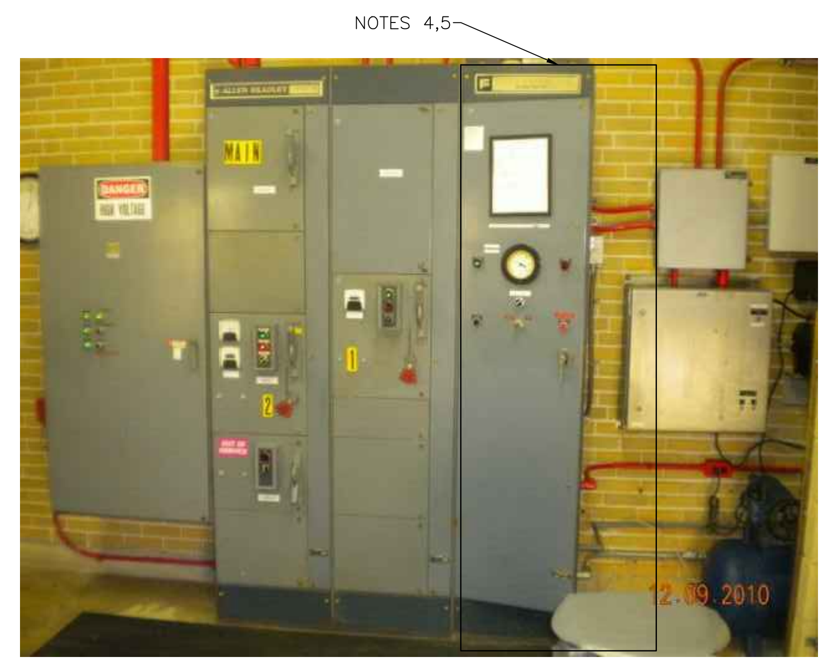
4 EXISTING CONTROL PANEL SCALE: NOT TO SCALE
