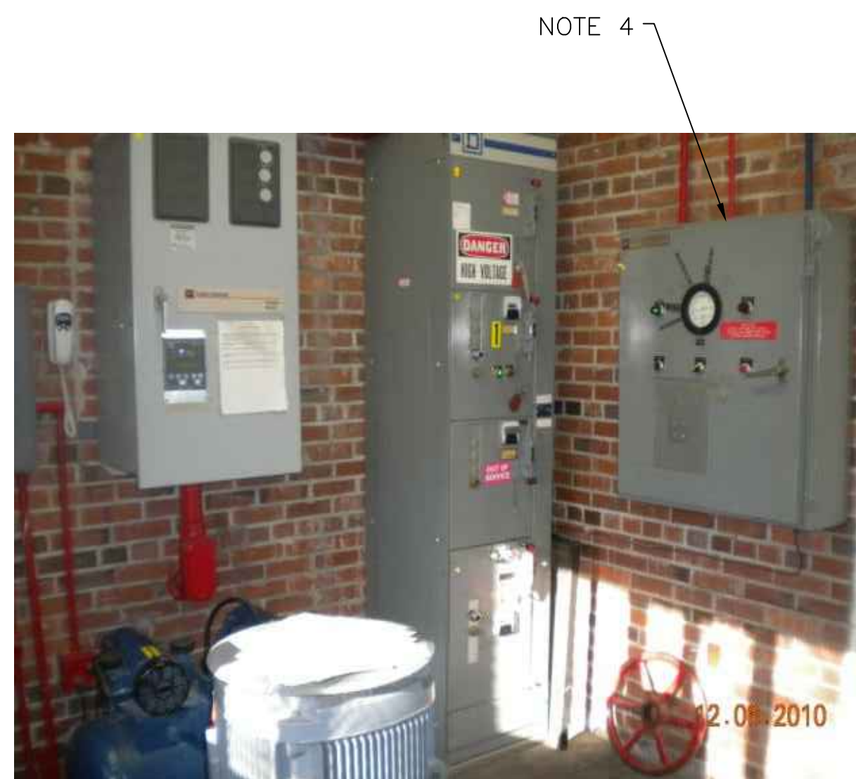
3 EXISTING CONTROL PANEL SCALE: NOT TO SCALE
