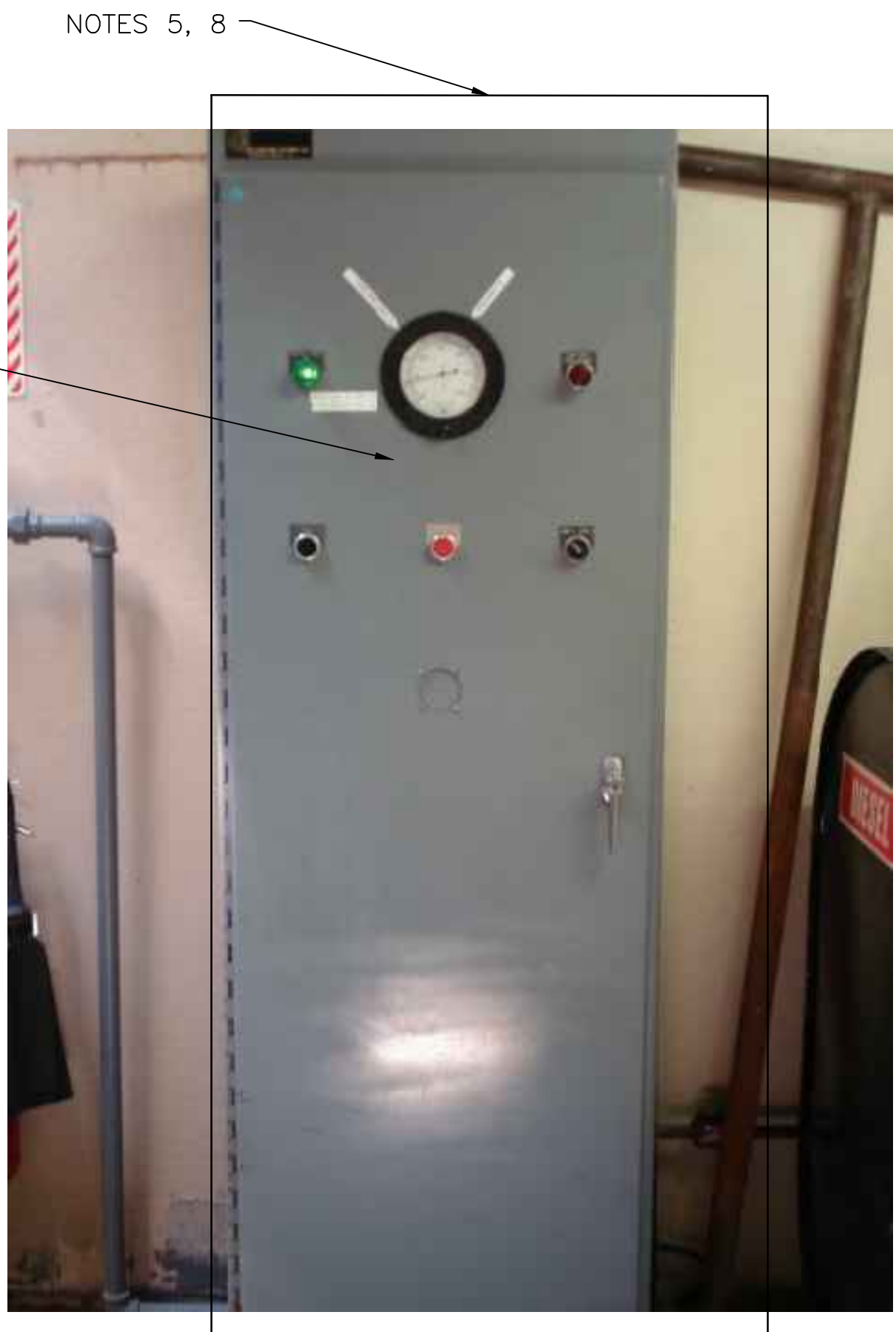
4 EXISTING CONTROL PANEL SCALE: NOT TO SCALE
