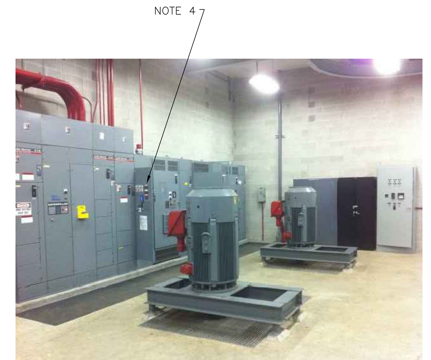
4 EXISTING CONTROL PANEL SCALE: NOT TO SCALE
