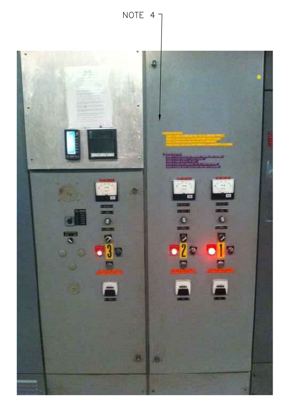
4 EXISTING CONTROL PANEL SCALE: NOT TO SCALE
