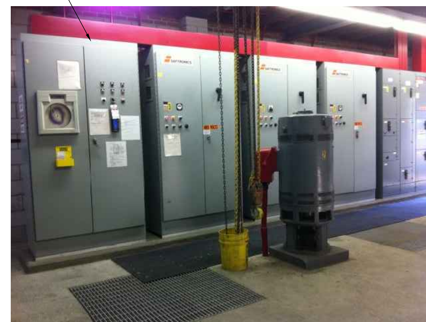
3 EXISTING CONTROL PANEL LOCATION SCALE: NOT TO SCALE
